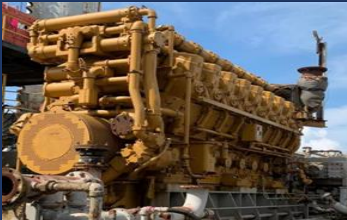
Caterpillar Gas Generator
