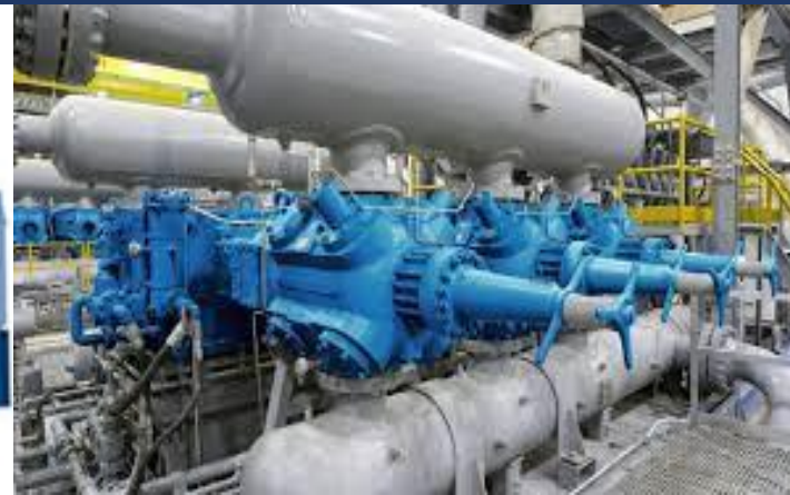
Ariel Gas Compressor
